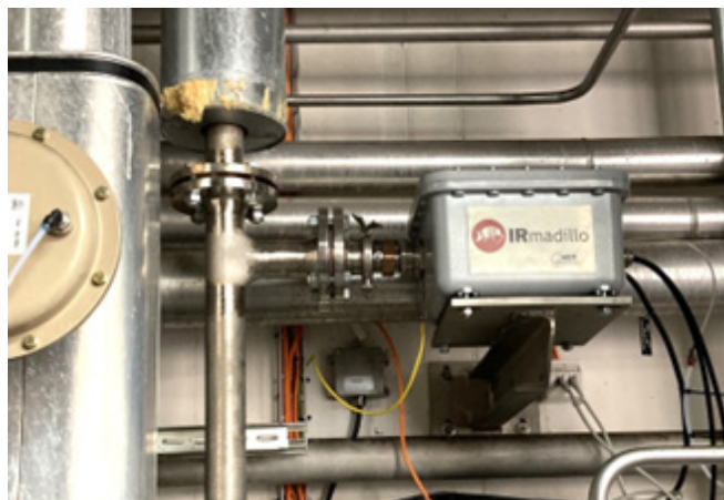
Figure 1: IRmadillo installed on the inlet of the centrifuge upstream of caustic addition.
